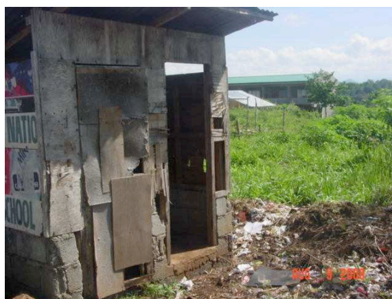
This old toilet is for 305 students of Balubal National High School
