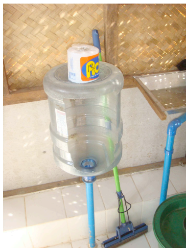
Inside an Ecosan UDD Toilet, 5 gallon plastic bottles are innovatively transformed into urinals
